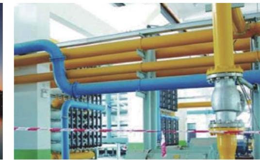
Daishan County Xiushan Seawater Desalination Project
